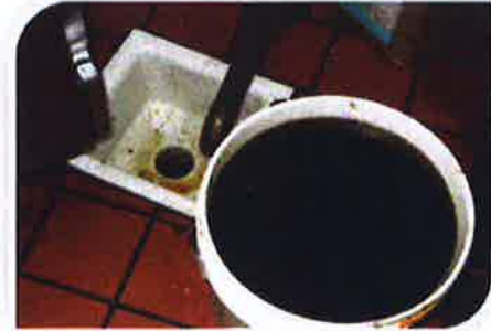
A Kitchen BMP Violation is Identified During Inspection
