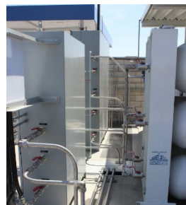
Matrix Valve Panel and Priority Valve Panel
