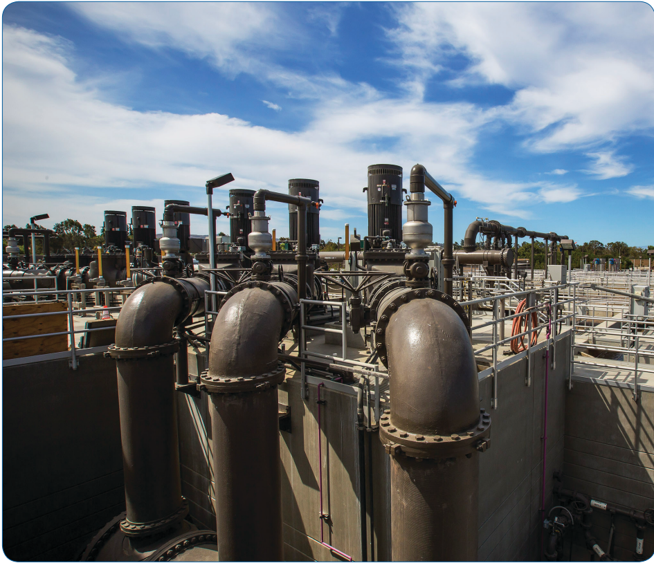
Pumps and pipes for the membrane bioreactor at the expanded Michelson Water Recycling Plant.
