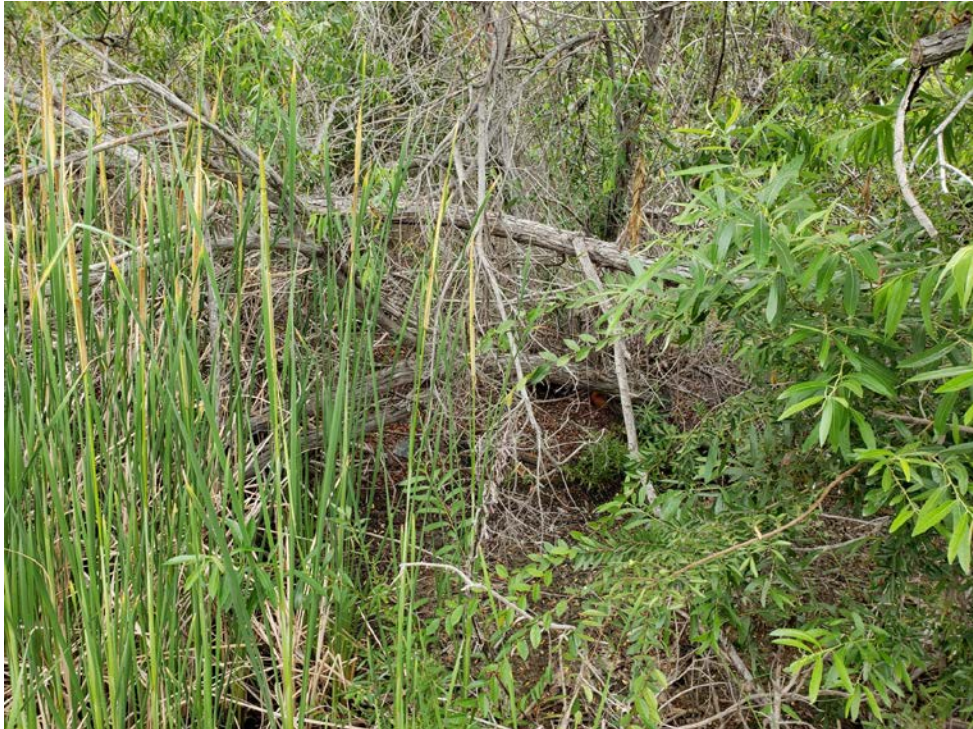
The outlet exit portal is obstructed and the surrounding area needs to be cleared.
