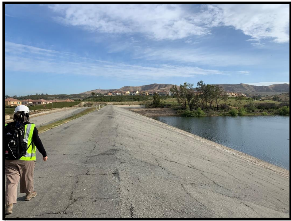
Photo 2) AC-lined crest and upstream face. Note cracks.
