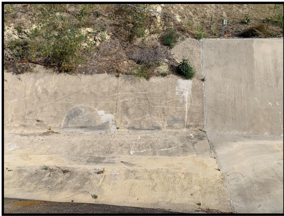
Photo 10) Recent spillway channel repairs. Note vegetation growing at top of wall.
