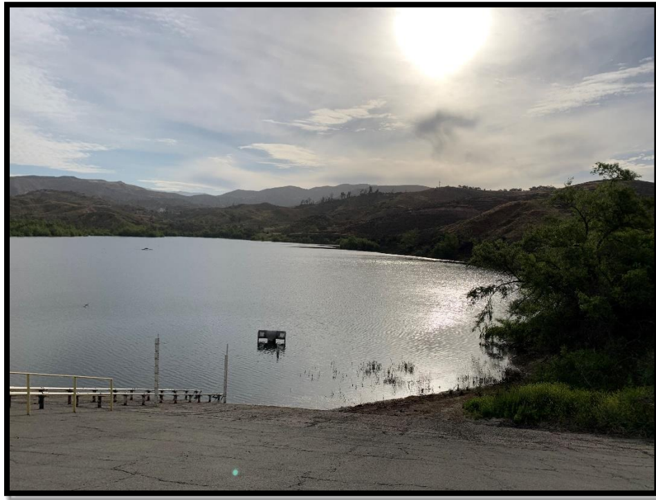
Photo 1) Left end of AC-lined upstream face and the reservoir. Note the screened outlet intake and encroaching vegetation on groin area.
