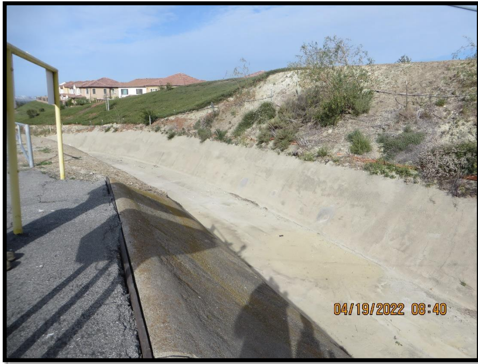
Photo 9) Spillway channel looking downstream from end of dam crest. Note separation between AC pavement and spillway concrete liner joint.
