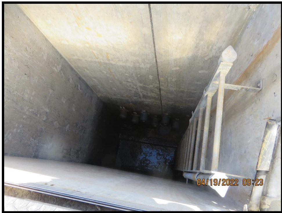
Photo 14) Seepage drain-pipe outfalls at the bottom of the seepage vault downstream of dam.
