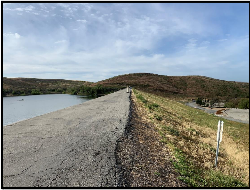
Photo 3) AC-paved crest with cracking and low grass cover on downstream face looking towards left abutment.
