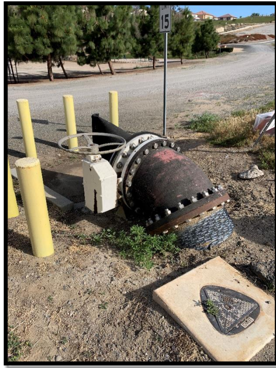
Photo 13) 24-in-diameter butterfly blowoff valve looking downstream.
