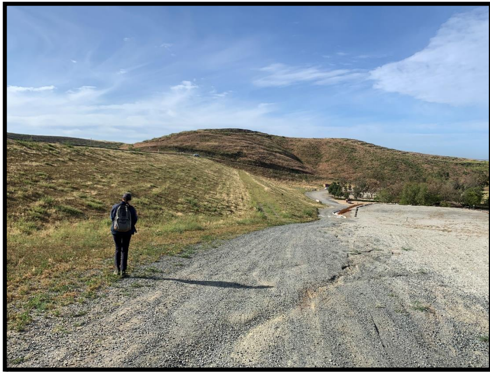
Photo 6) Downstream face looking towards left abutment. Note rill erosion on access road.
