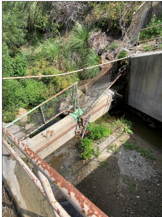
Photo 15) Looking downstream at the energy dissipator structure and exit channel, note vegetation encroachment.
