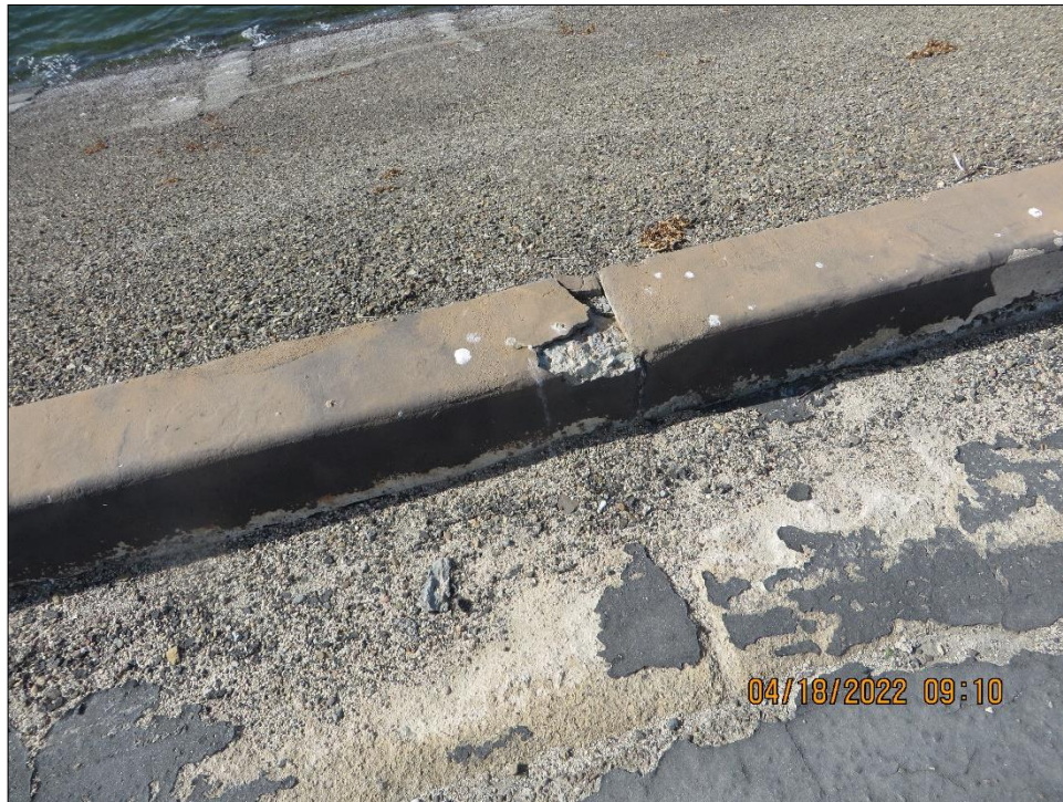
Photo 7) Cracking and spalling at joints of concrete crest curb on upstream side.
