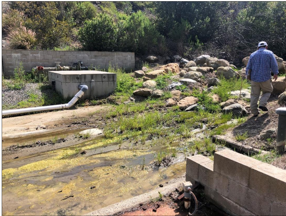
Photo 22) Toe and Floor Seepage Concrete Vault with wet toe area.
