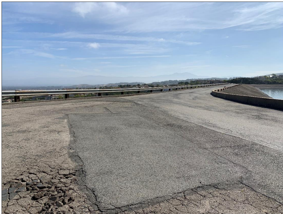
Photo 6) AC paving cracking near left abutment area.
