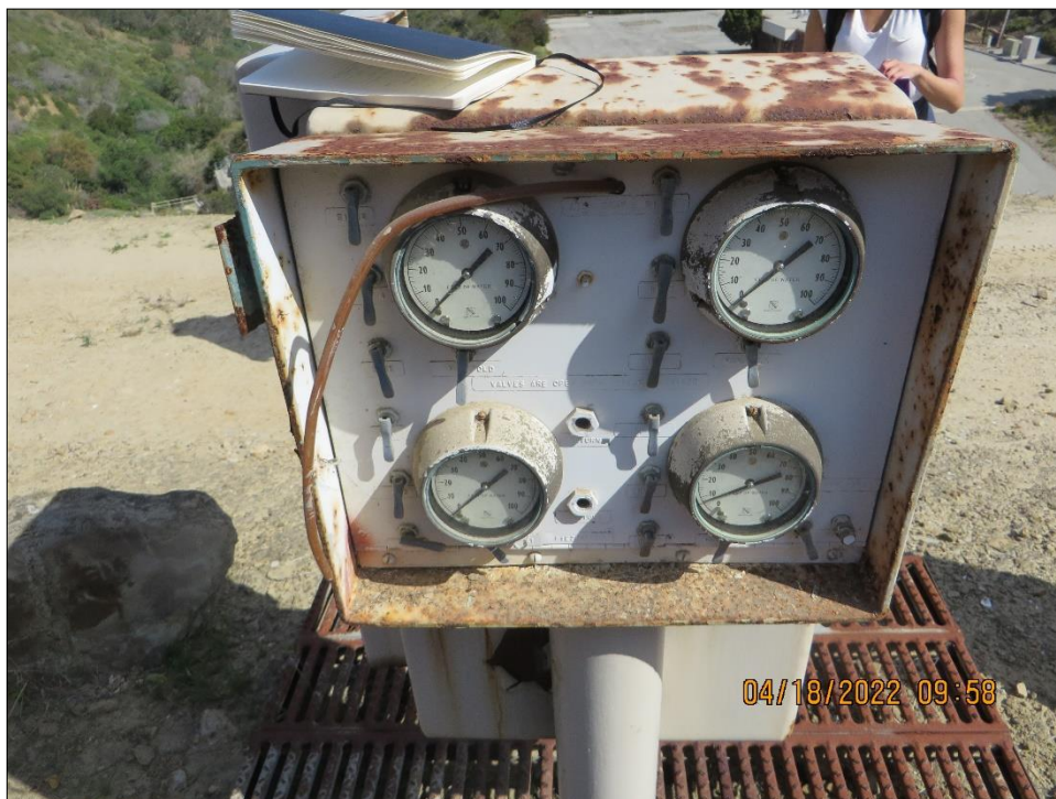
Photo 23) Corroded pneumatic piezometer gauge box.
