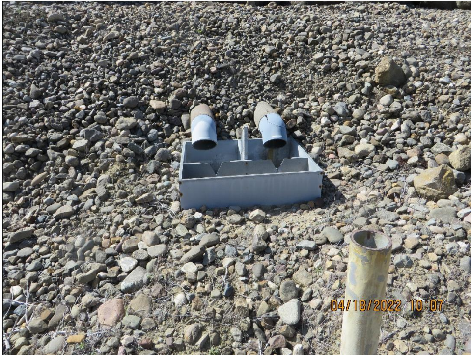
Photo 18) V-notch weirs measuring seepage flows from the Upstream Collector Drains #1 and #2.
