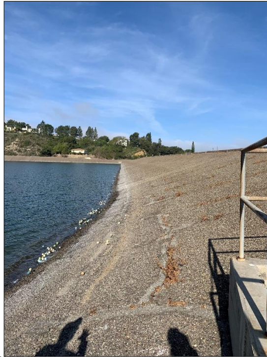
Photo 3) View of upstream AC liner cracking and edge of right spillway drop inlet
