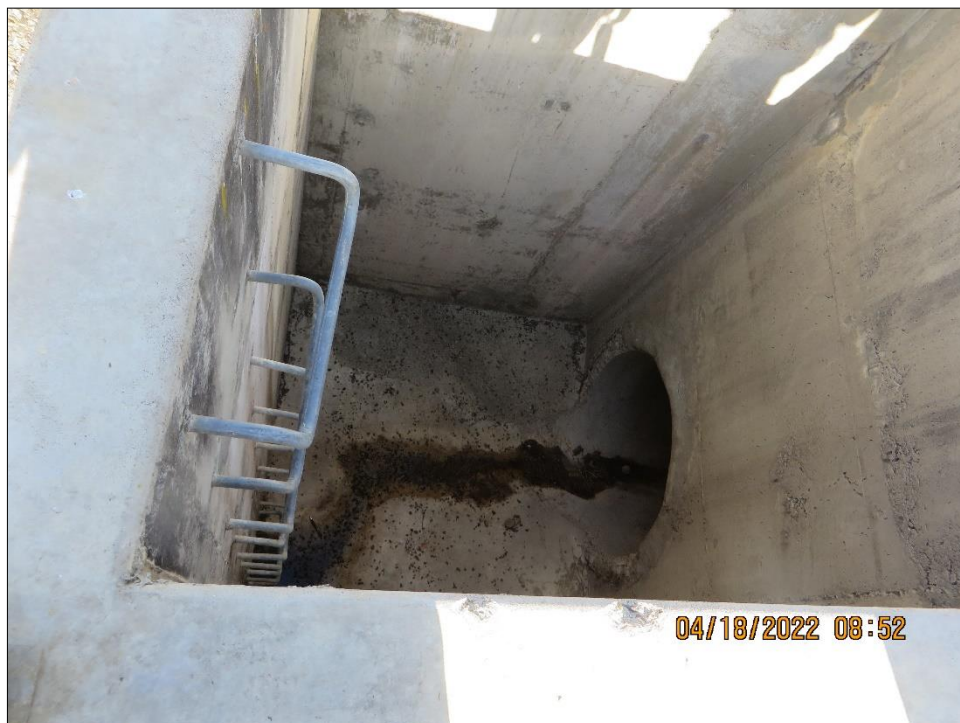
Photo 13) Bottom of right spillway drop inlet structure leads to a 48-inch spillway pipe that discharge at the dissipator structure located at the downstream toe of the dam.
