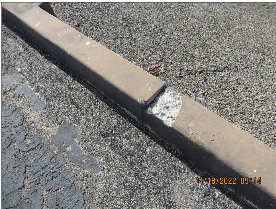
Photo 8) Cracking and spalling at joints of concrete crest curb on upstream side.
