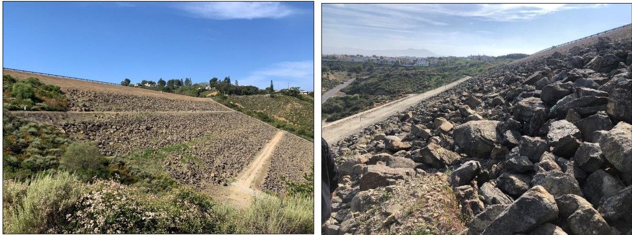
Photo 9) Downstream face looking towards the left abutment and the right abutment, respectively.
