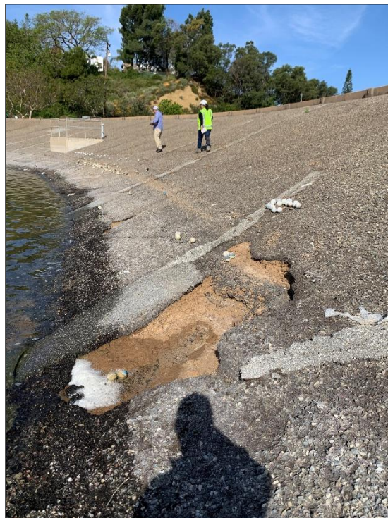
Photo 4) Significant AC liner pothole at left side of upstream face. Note left spillway drop inlet.
