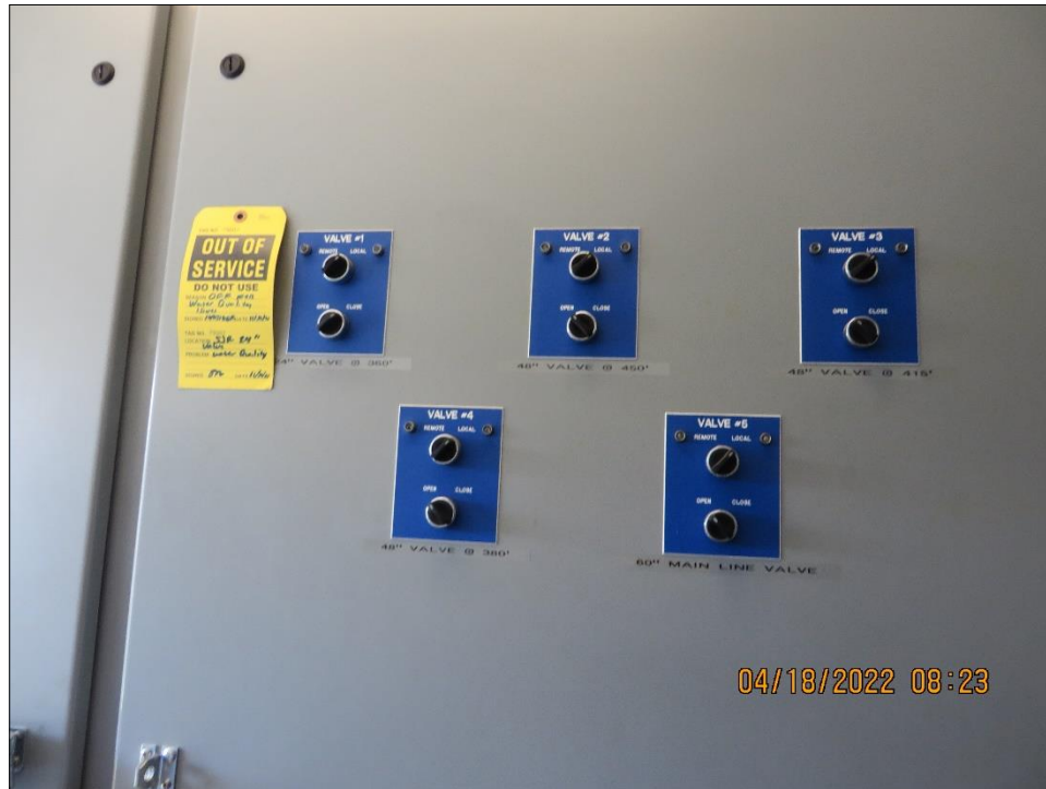
Photo 16) Outlet valve control panel door at the reservoir control room.
