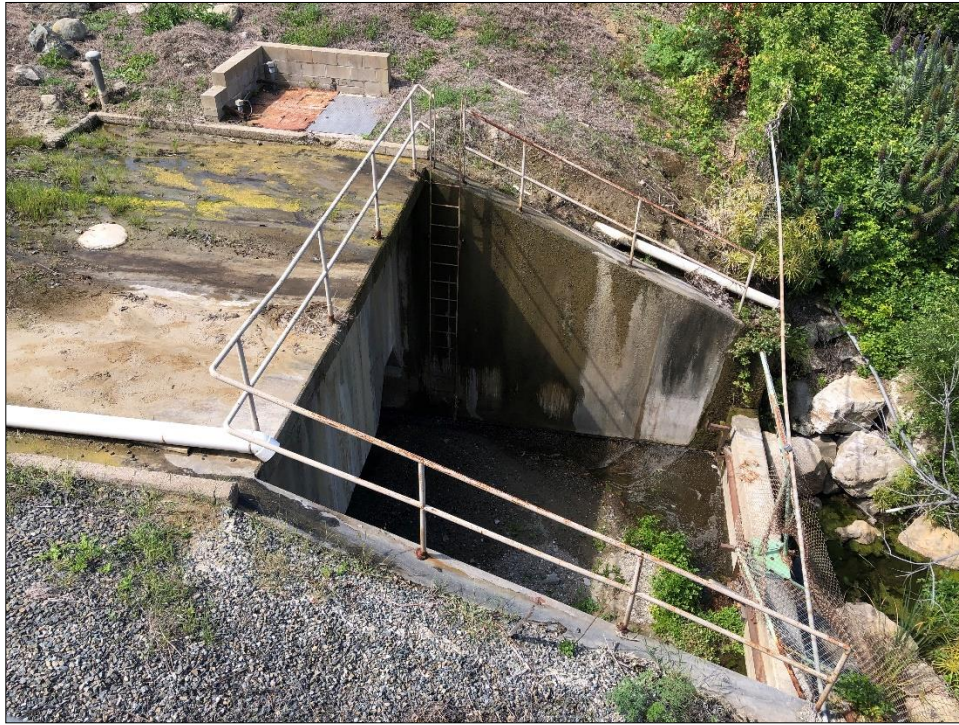
Photo 14) Energy dissipator structure with minor normal seepage coming from dam toe.
