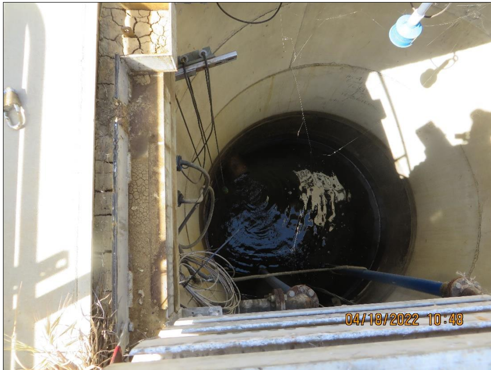
Photo 20) Inside view of East, West, Filter drains seepage collection vault.
