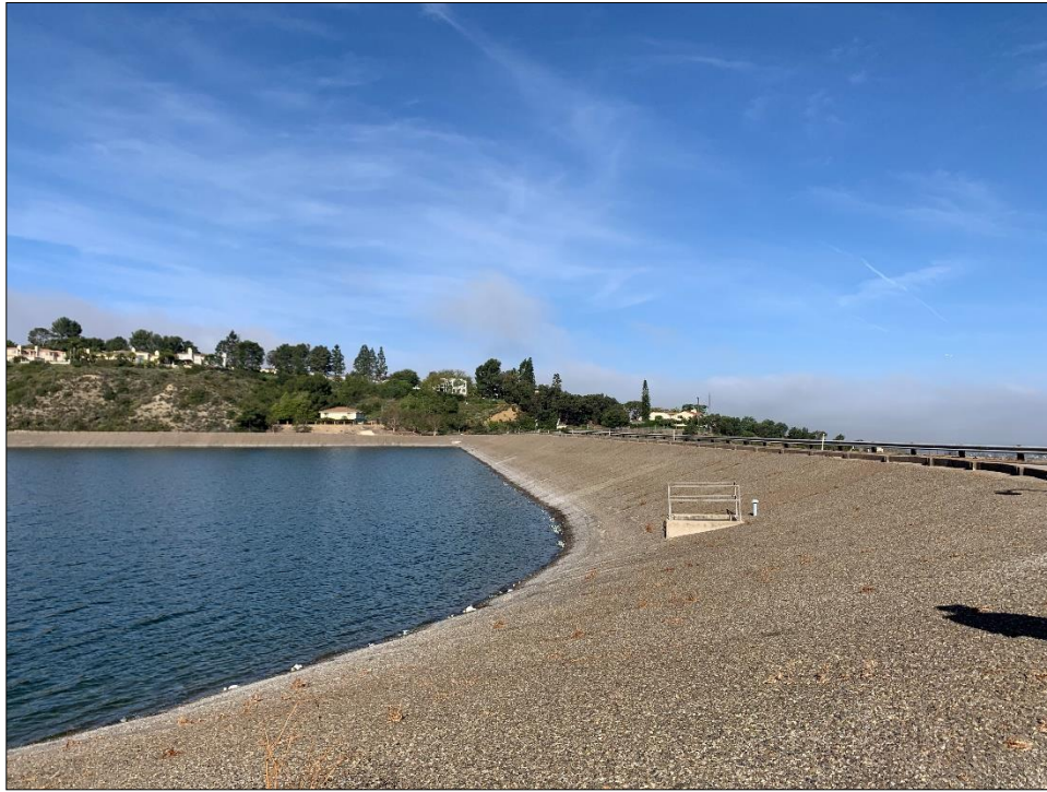
Photo 1) AC-lined upstream face looking towards left abutment. Note two spillways drop inlets.
