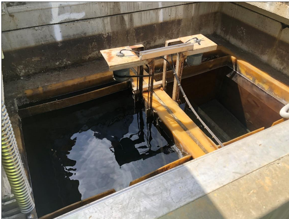
Photo 17) V-notch weirs located near the energy dissipator structure, measuring seepage from the Toe and Floor Drains.
