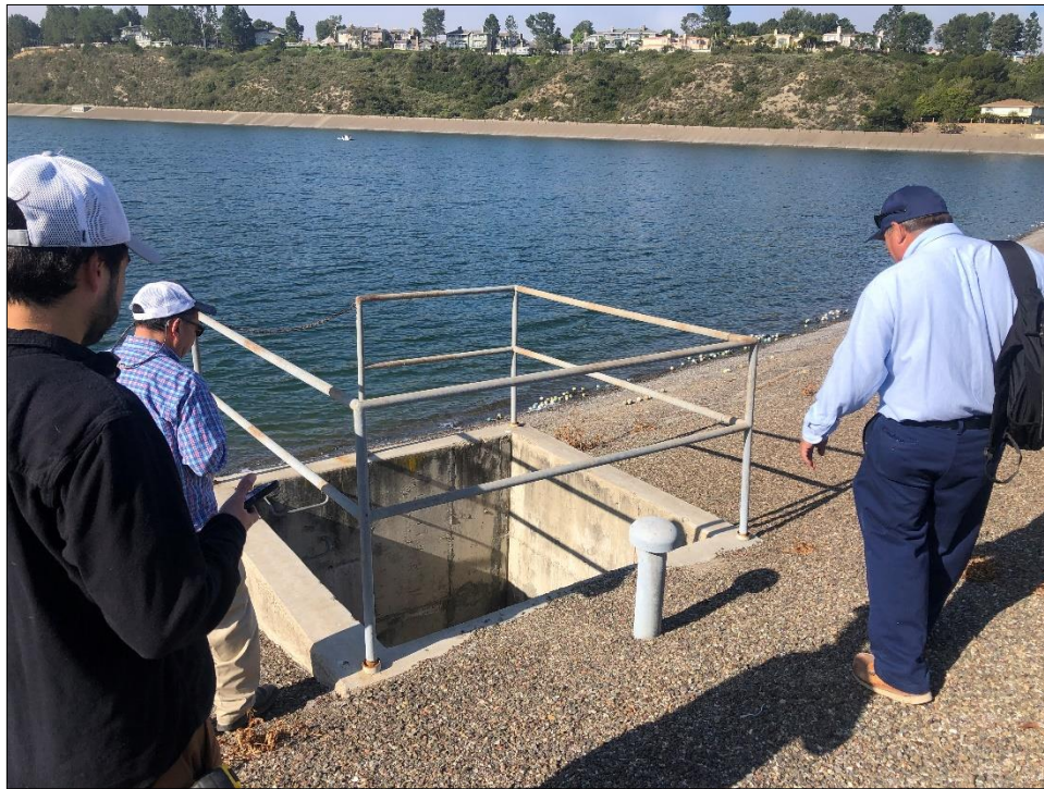
Photo 12) Close up of one (right) of the two spillways drop inlet structures located at upstream side of dam.
