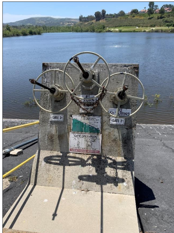
Photo 12) Outlet upstream valves' operating equipment.
