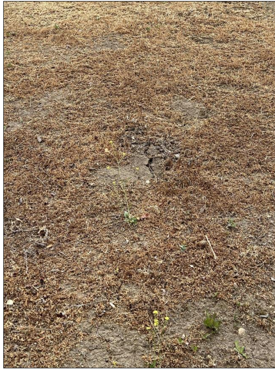
Photo 17) Soil desiccation cracking near piezometer P-7. Photo taken by IRWD on 6/13/2022 DSOD inspection.
