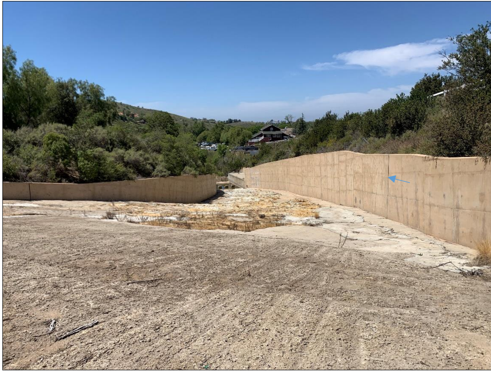
Photo 9) Spillway channel looking downstream, note vertical right wall joint offset.
