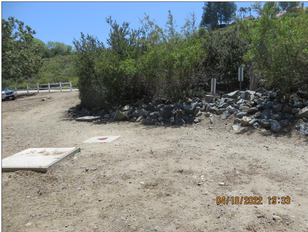
Photo 14) Location of downstream outlet control valves.
