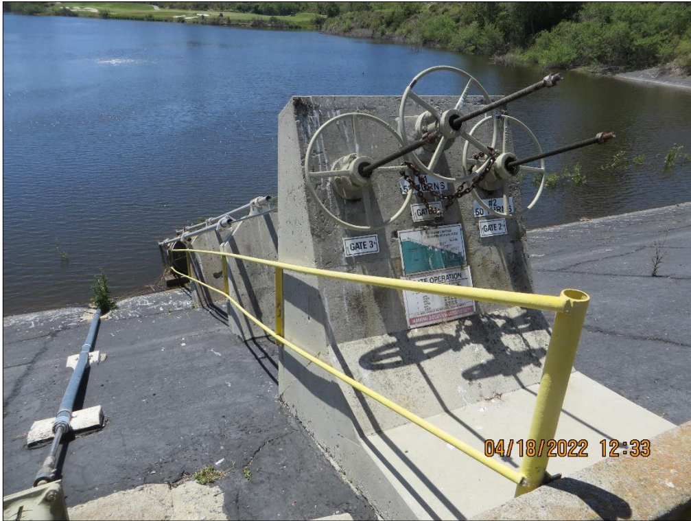
Photo 13) Outlet valve controls and stems.
