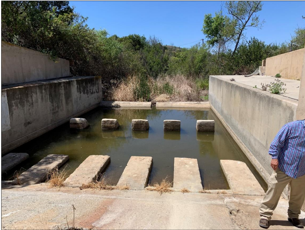
Photo 11) Close up view of spillway stilling basin, note brush/tule growth downstream.
