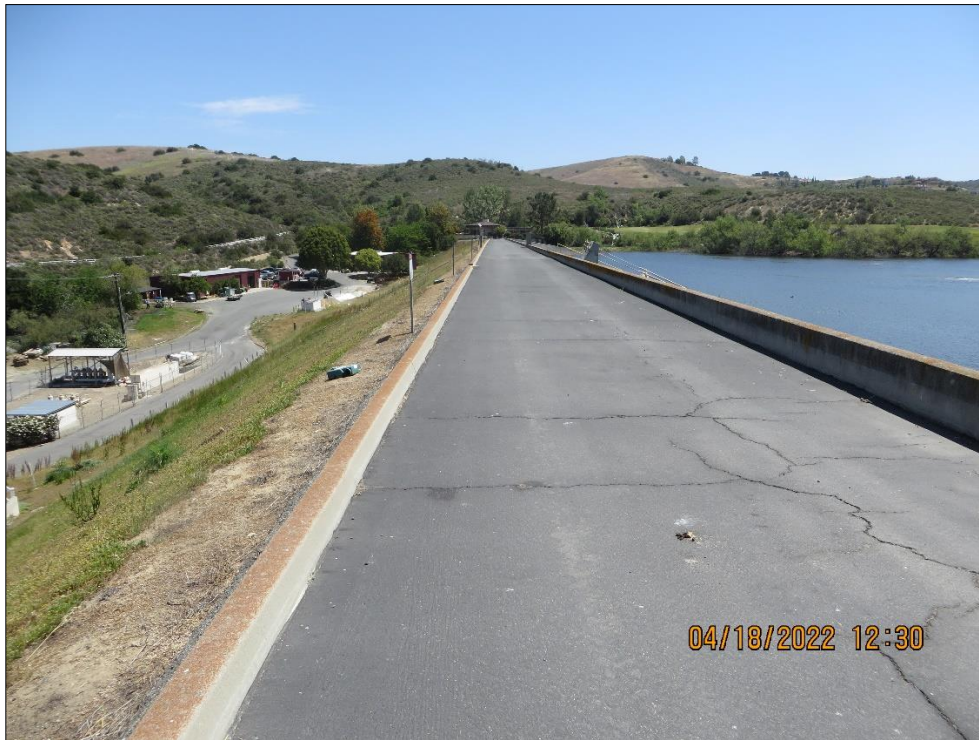
Photo 3) Minor AC paving temperature related cracking looking towards the right abutment.
