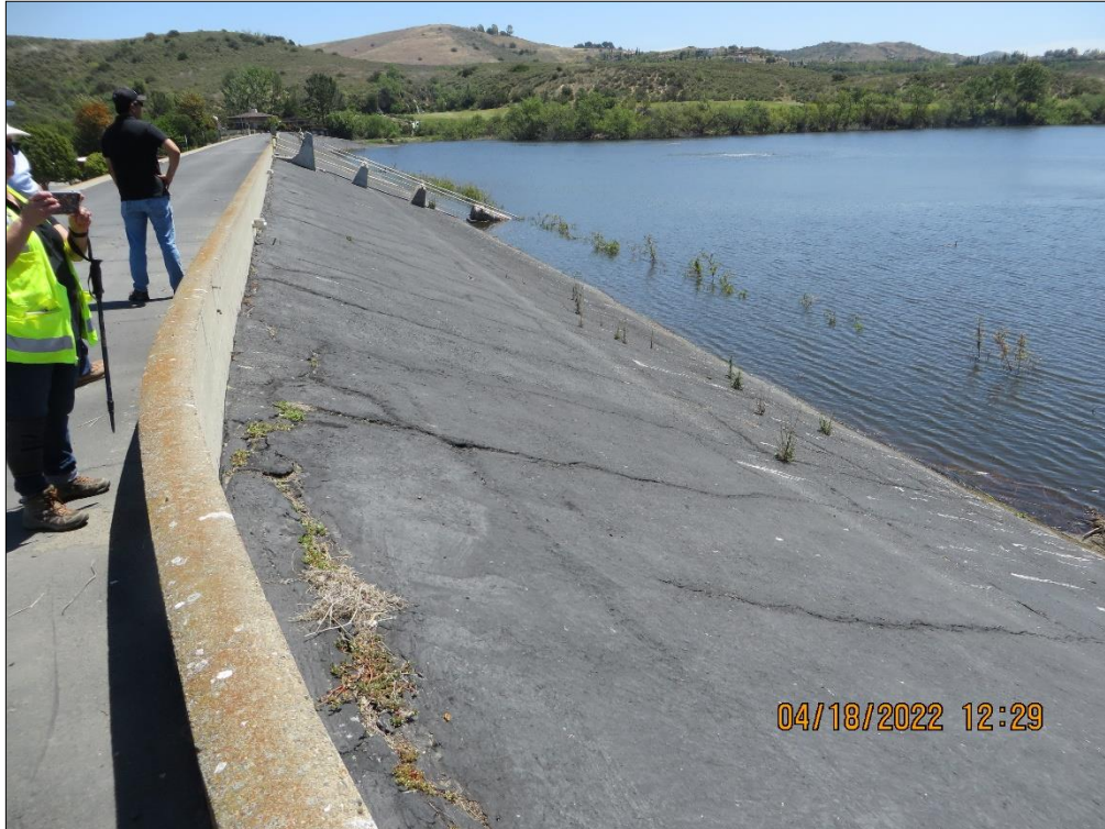
Photo 4) AC-lined upstream face looking towards right abutment. Note cracks and brush in reservoir.
