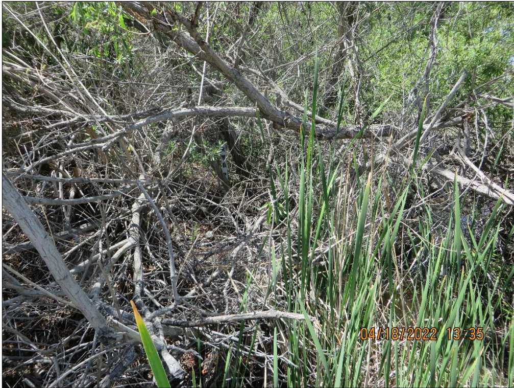
Photo 15) Overgrown vegetation at 30-inch blowoff discharge outfall.
