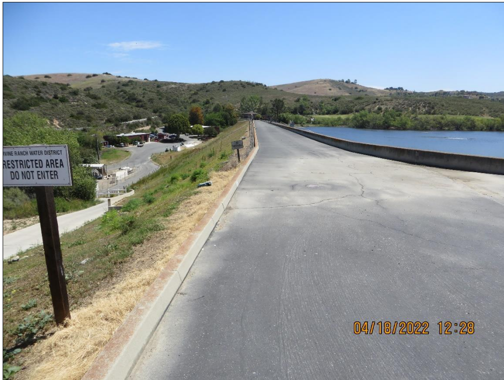
Photo 2) Minor AC paving cracking near left abutment looking towards the right abutment.
