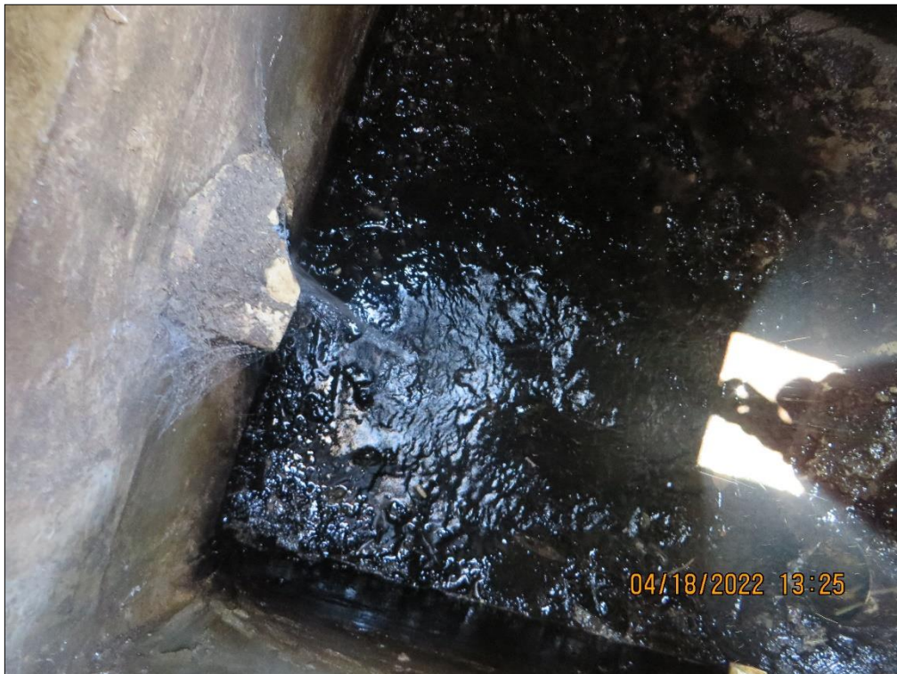
Photo 16) Seepage at left subdrain.
