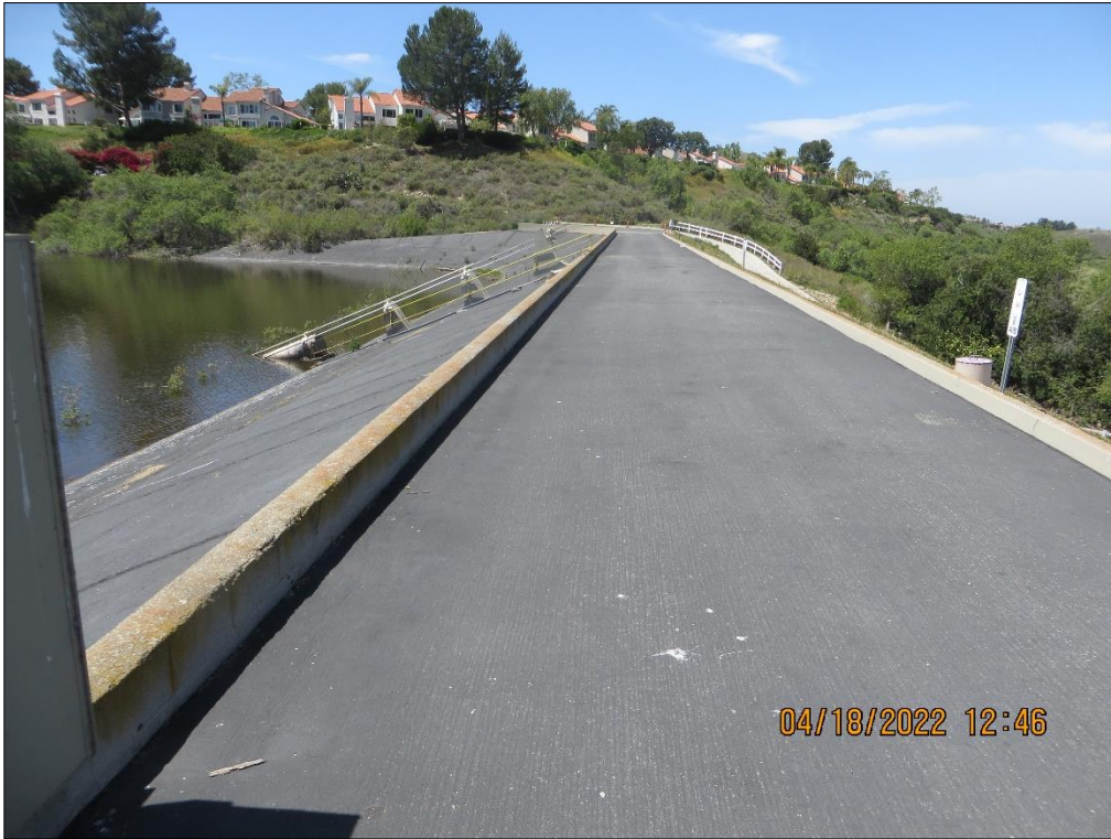
Photo 1) AC paved crest and upstream face looking towards the left abutment, including 1 foot-high curb wall.
