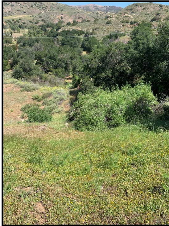
Photo 15) Downstream slope looking at right groin. Note overgrown vegetation.
