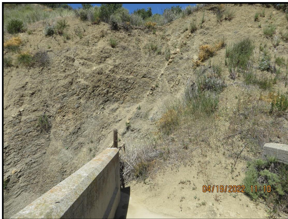
Photo 10) Close up soil debris sloughing from left abutment slope onto pedestrian bridge.
