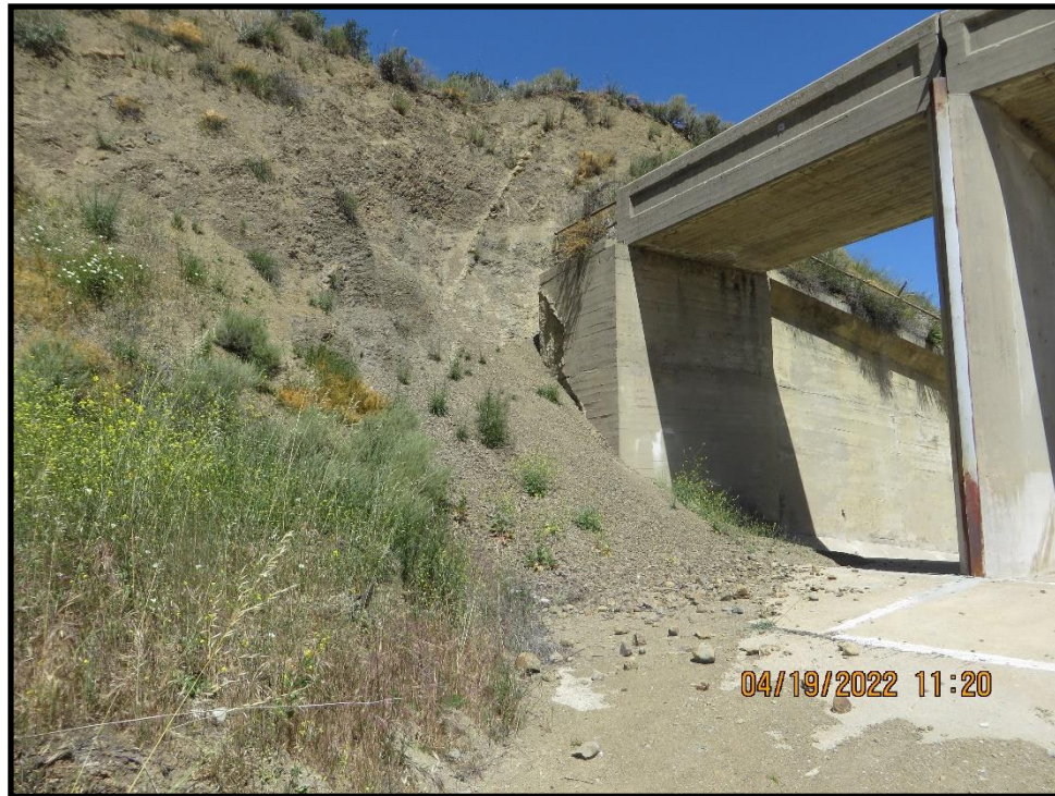
Photo 9) Overview of left abutment sloughing onto concrete approach.
