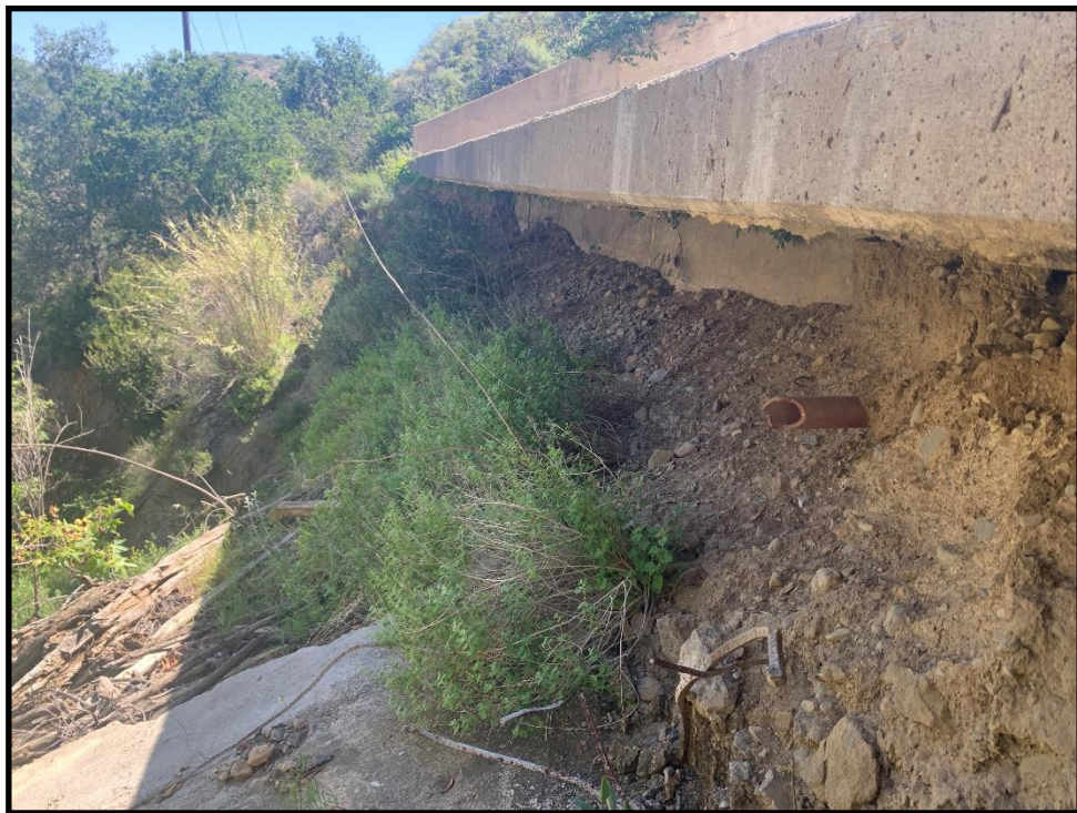
Photo 14) Undercutting/erosion at the downstream end of the spillway chute.
