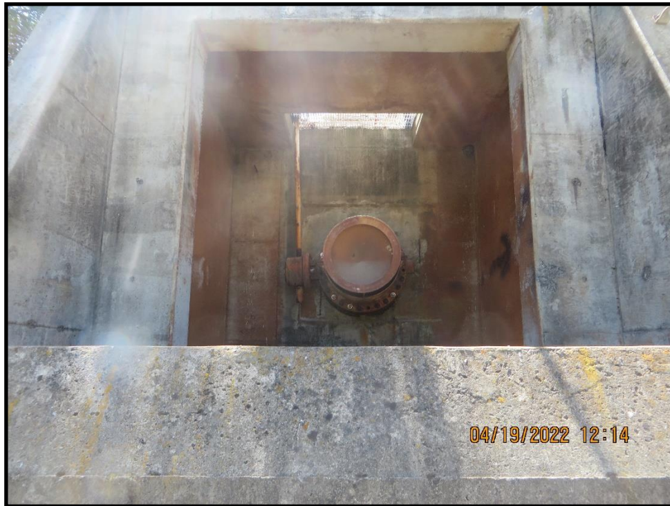
Photo 19) Emergency blowoff valve within dissipator structure.
