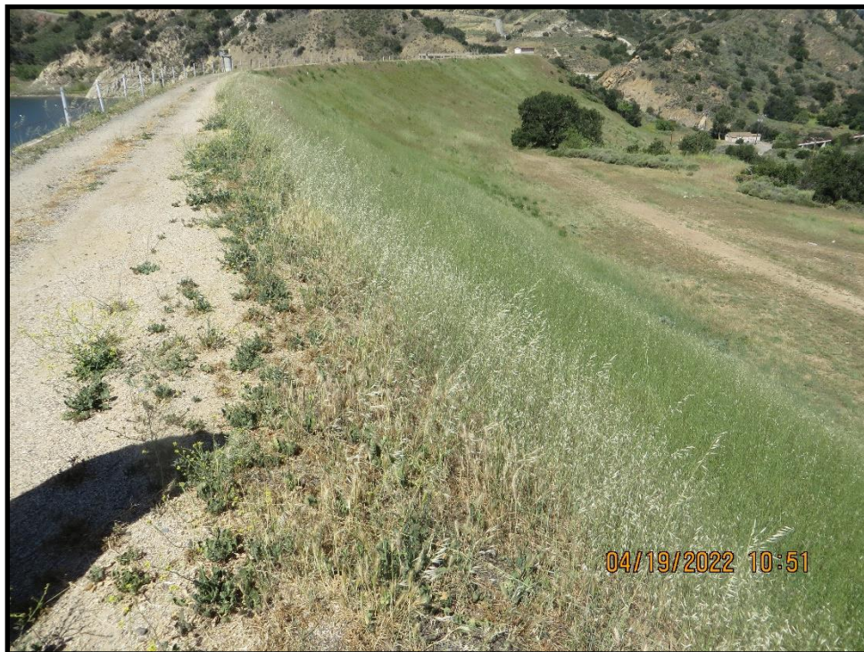
Photo 2) Crest and Downstream Slope looking toward main section of dam from right abutment area.
