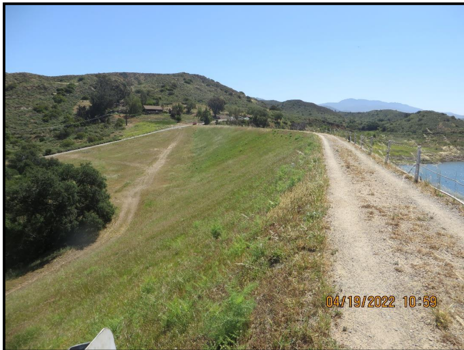
Photo 4) Crest and downstream slope looking towards right abutment area. Note vegetation near right groin.
