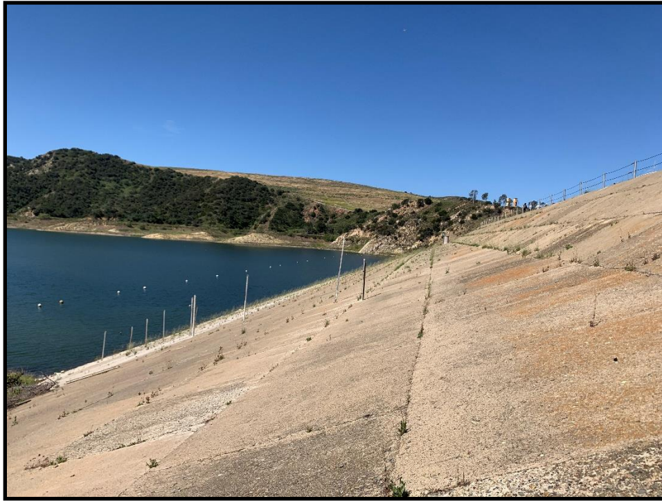
Photo 3) Upstream face looking towards left abutment. Note vegetation growing in cracks.
