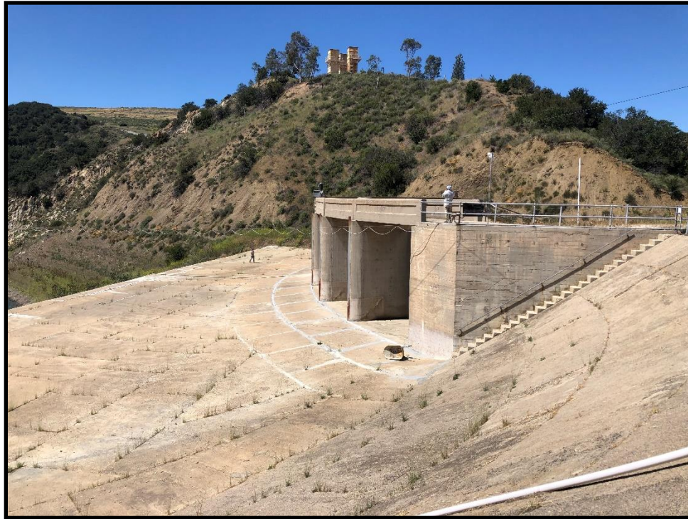
Photo 5) Left end of upstream slope of dam and spillway concrete approach looking toward left abutment.
