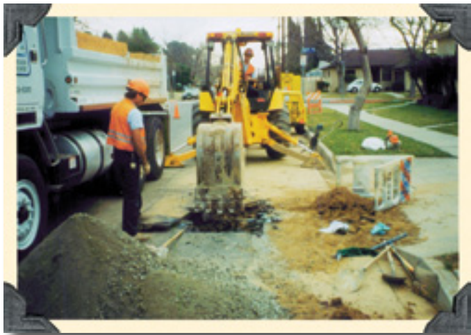
In 1994 IRWD crews rotated through 12-hour shifts over a four-day period to restore water to earthquake-damaged areas of Northridge and Reseda.
