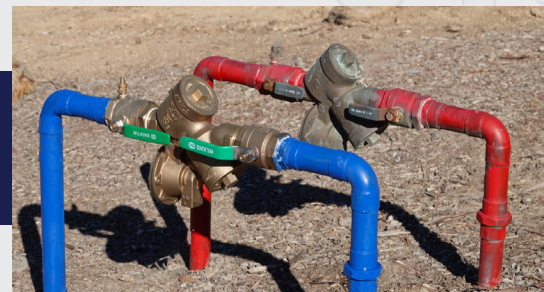
▲ Typical backflow devices
